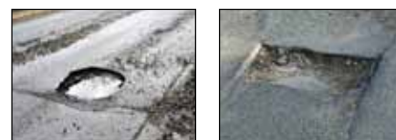
Photos 1 & 2 :Untreated Potholes
